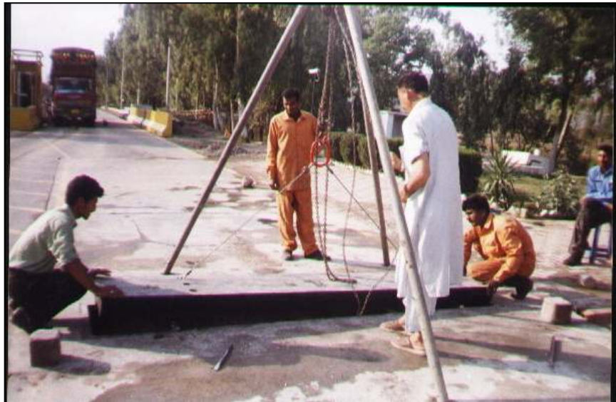
Slow Speed Weigh in Motion Scale (SSWIM) installation works, National Highway N-5
